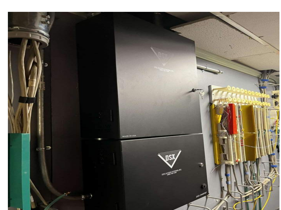
IMG_8273 SALVAGE IT EQUIPMENT @ TELECOM CLOSET IN MEDIA CENTER
