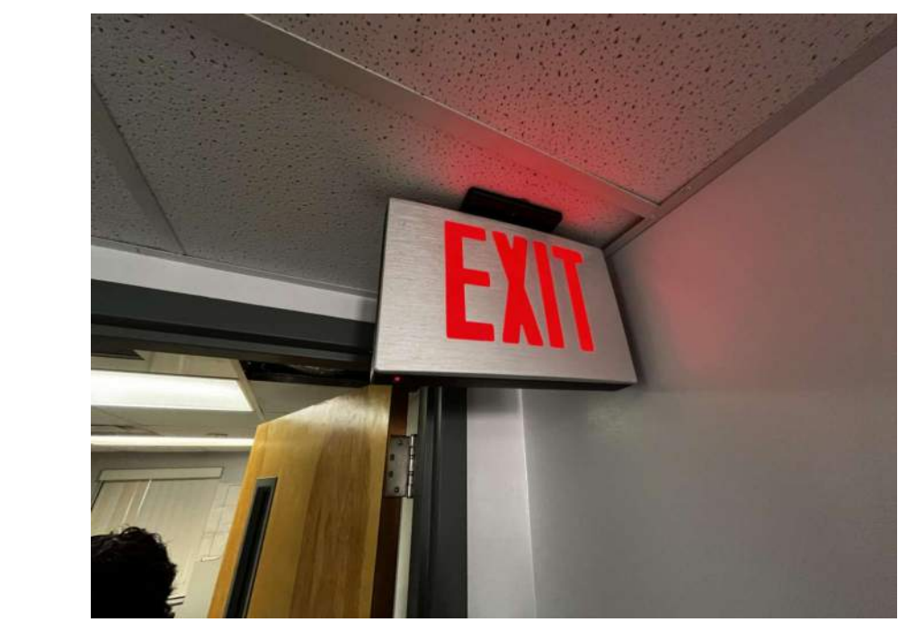
IMG_8281 SALVAGE ALL EXIT SIGNAGE
