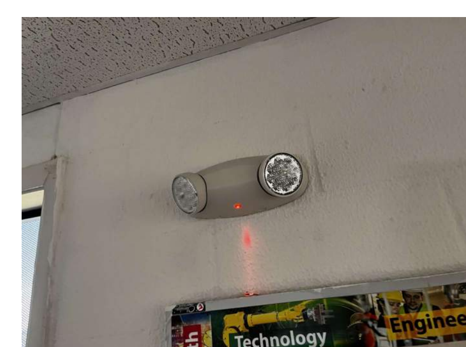
IMG_8269 SALVAGE ALL EMERGENCY LIGHT FIXTURES
