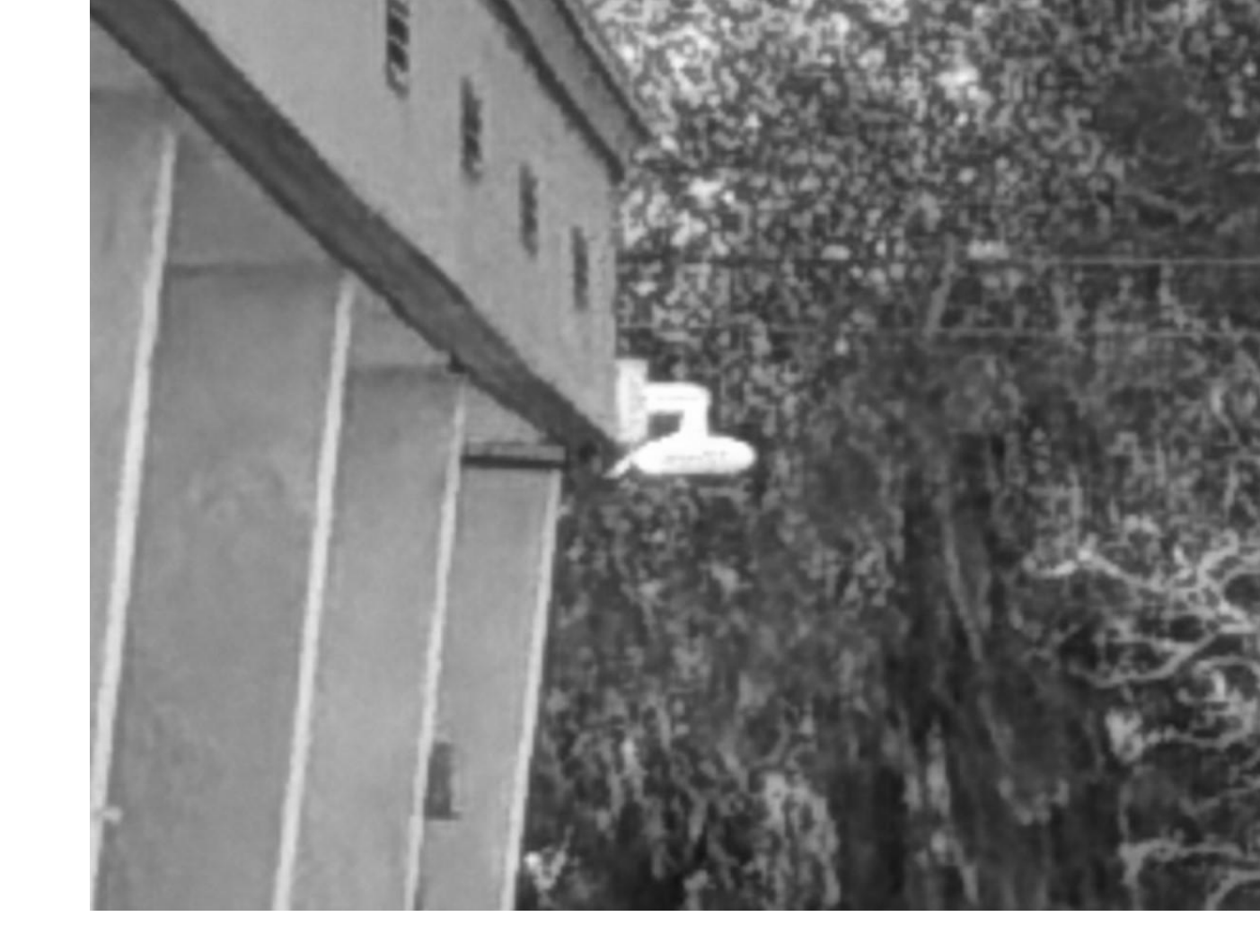
13 - EXTERIOR SECURITY CAMERAS
