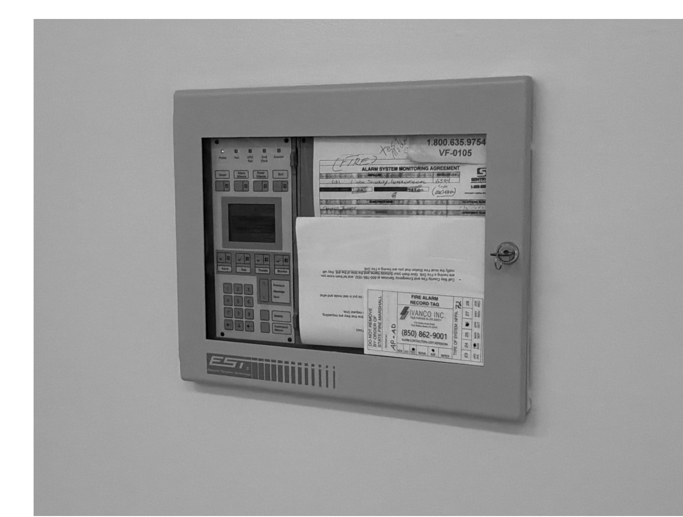
6 - FIRE ALARM ANNUNCIATOR PANEL
