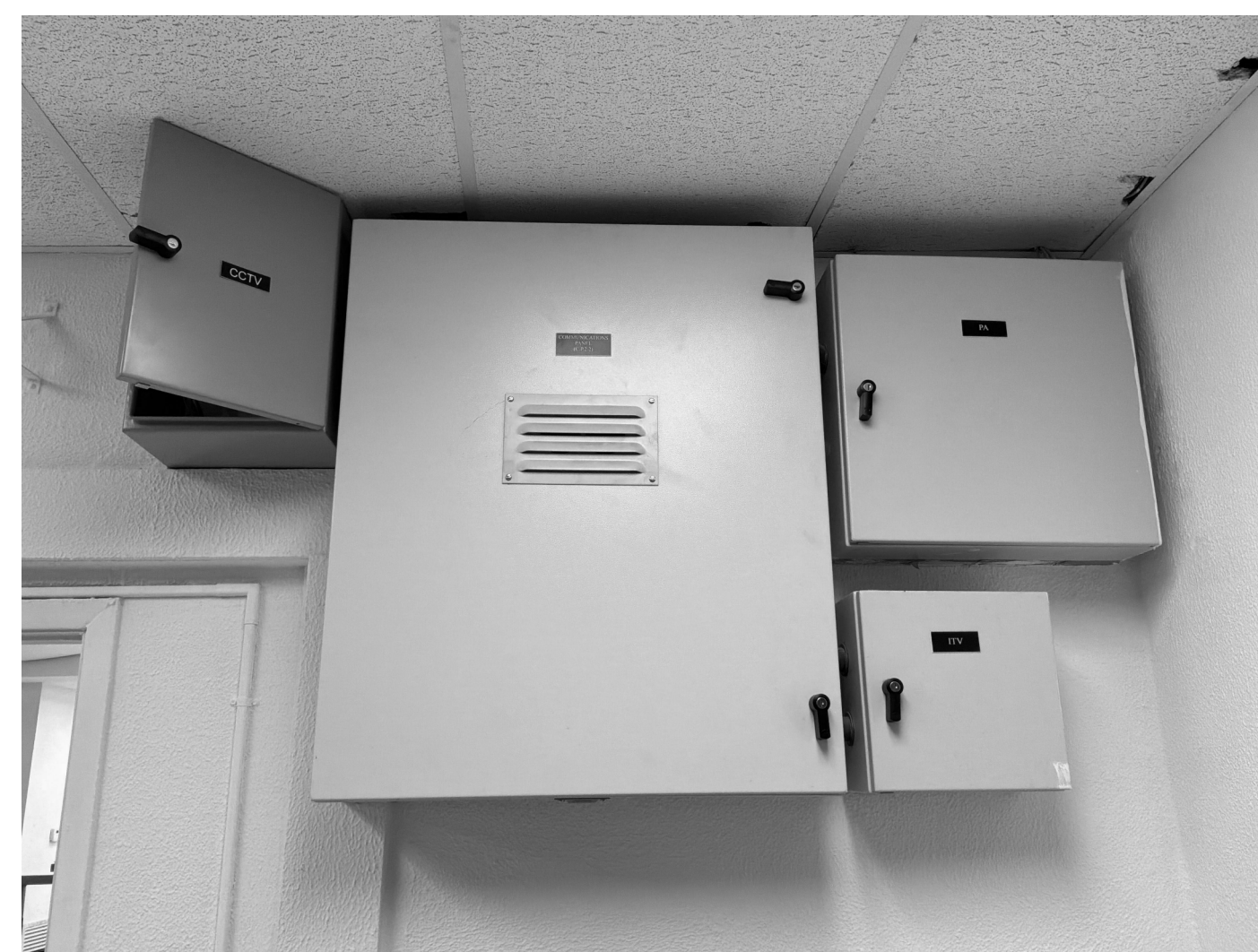
2 - COMMUNICATIONS, CCTV, PA, ITV PANELS
