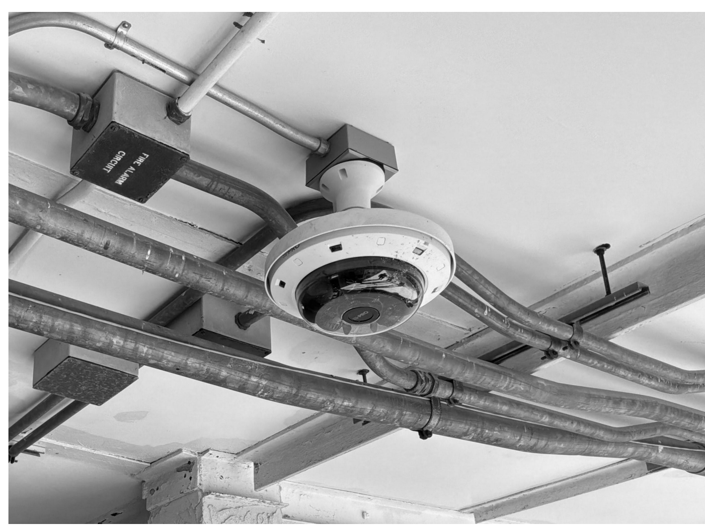
11 - COVERED WALKWAY SECURITY CAMERAS
