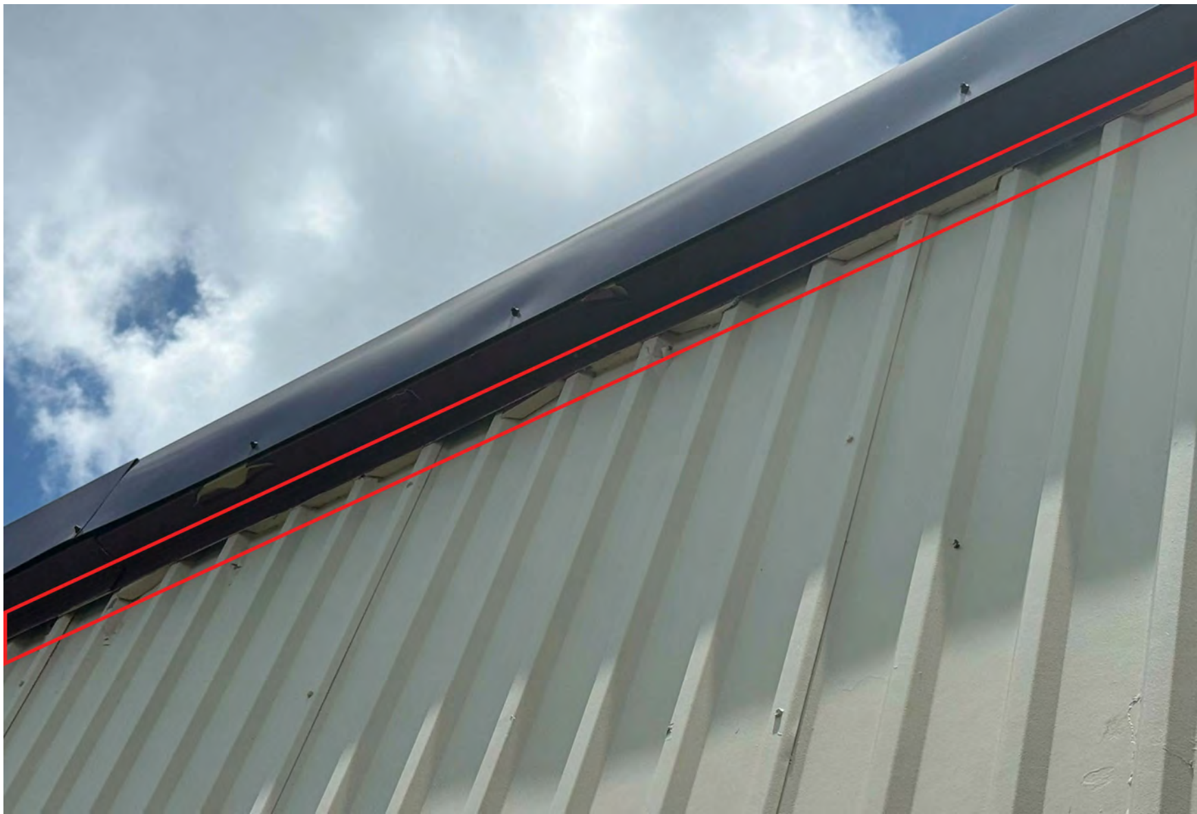
PHOTO OF EXISTING RAKE CONDITION:
